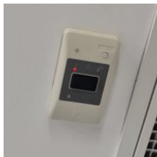
AC unit receiver (ON - red light lit)
