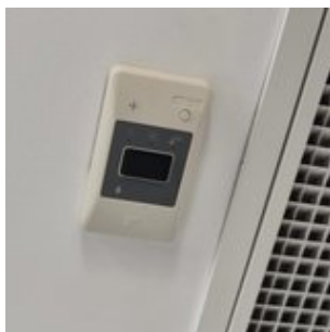
AC unit receiver (standby - no light)
